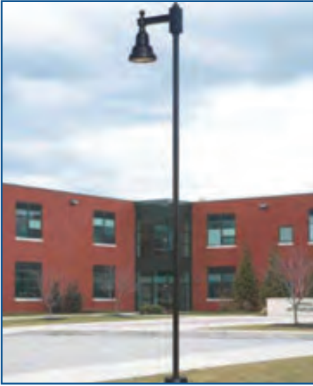
Alternative down casting lighting fixture along major street
